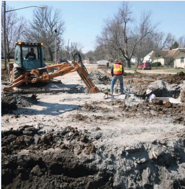
Crews have worked through the spring to get water main and storm drain construction complete on the Santa Fe Road Project.
